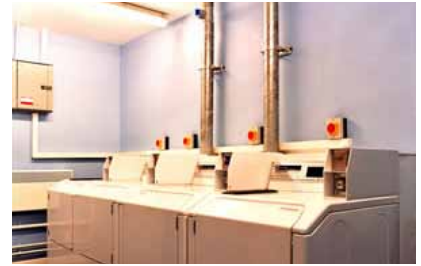
Laundry room at Sebastian Street
